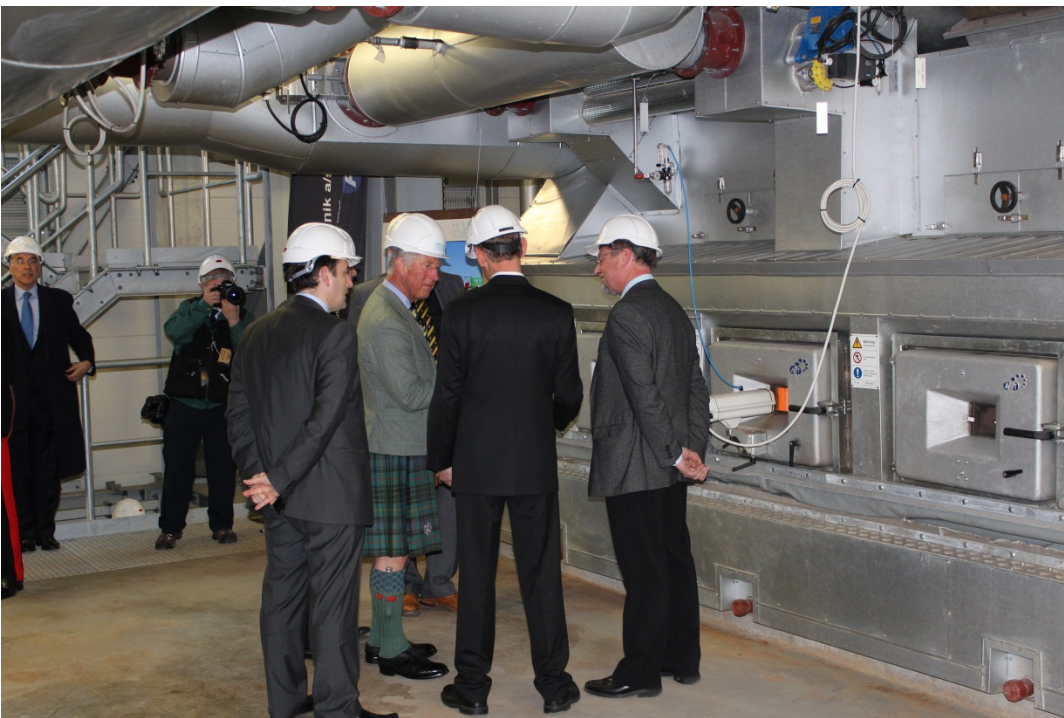
(Photo: HRH Prince Charles, Duke of Rothesay, Hans Erik Askou (CEO at AET and Torben Helge (Project Manager at AET) in front of the biomass fired boiler at the official opening of the Helius-CoRDe plant in Scotland)
